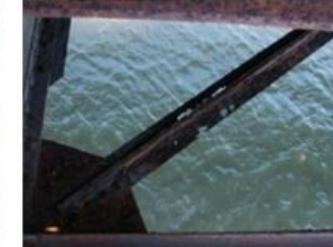
Loss of material
